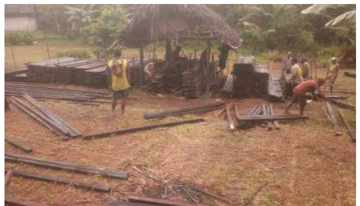
(above)The Locals at Yaputawe Village (Maposi) pilling the timbers for their new health centre building.
